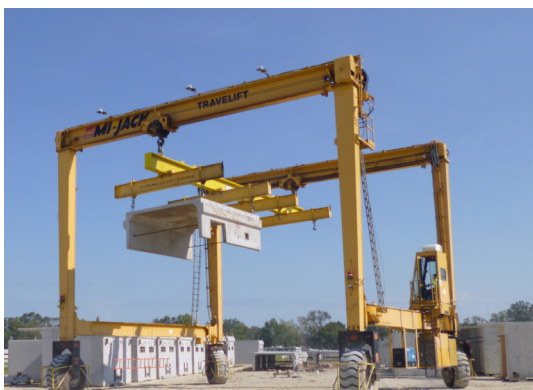
Plenum being transported to finish area
